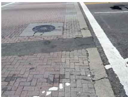
Decorative crosswalk treatments made of distinctive materials can become uneven over time (Credit: Ryan Snyder)
