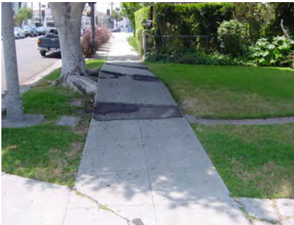
Uplifted sidewalk (Credit: Ryan Snyder)
