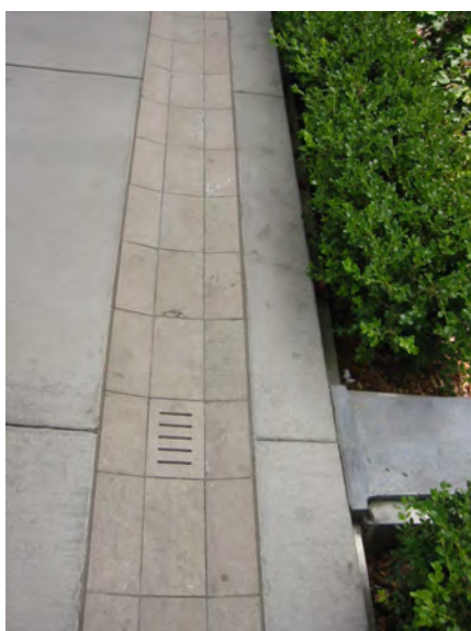
Constructed swale with drain (Credit: Stephanie Landregan)
